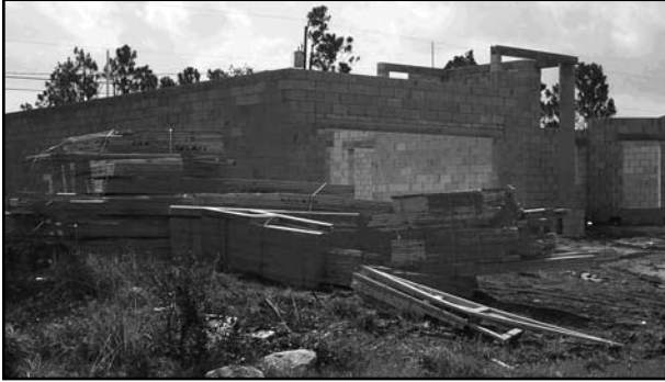
Example of large scale building materials being left unprotected during the early stages of a construction site.
