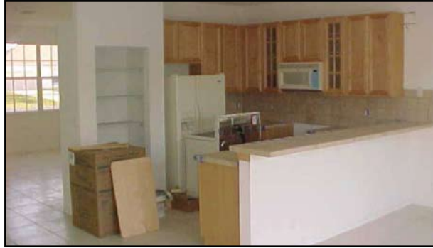
In this house under construction, the front door was left wide open with appliances left uninstalled in the kitchen.
