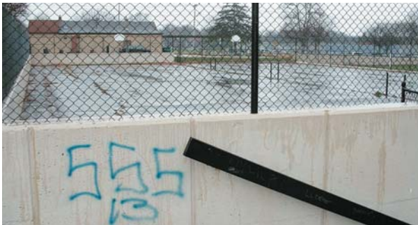
Graffiti tagging and other forms of defacement often mark school buildings and grounds.
