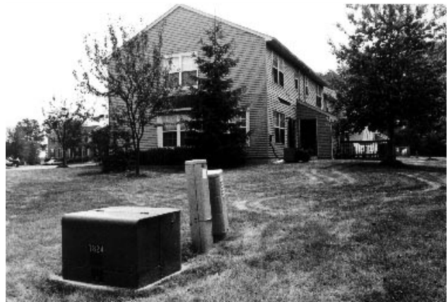
Malfunctioning electrical equipment may produce a steady pure tone that is best measured with an octave band analyzer. The Model Noise Ordinance and the State's Noise Control Regulations both regulate pure tones more strictly than mixed tones, as pure tones are generally regarded as being more annoying.
