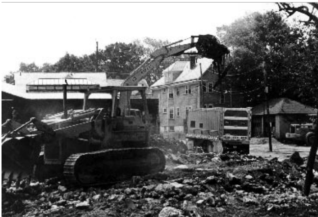
Construction and demolition may be curfewed by the adoption of VI(B)3.
