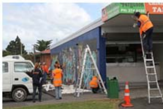
Manukau Beautification trusts working hard painting out the graffiti at the shops.
